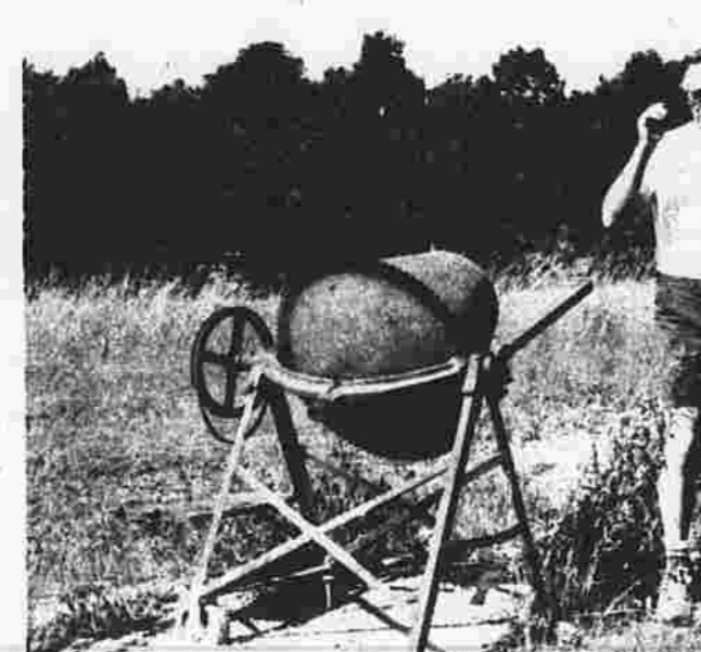
The Hursts stand by a cement mixer on the site of their proposed stand.
